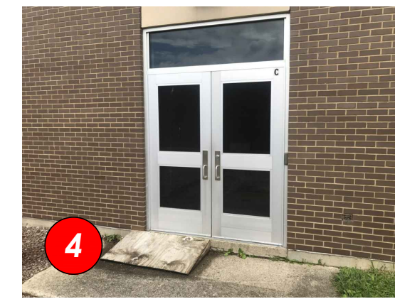
PROVIDE TWO NEW EGRESS RAMP AT EXTERIOR DOORS FOR A.D.A. ACCESS TO COURTYARD
